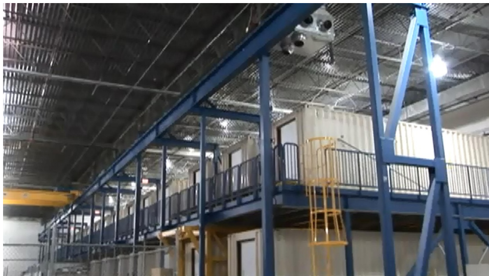
Figure 5: Google prefabricated modular data center 13
